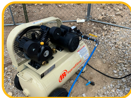
MaxLine attached to air compressor
