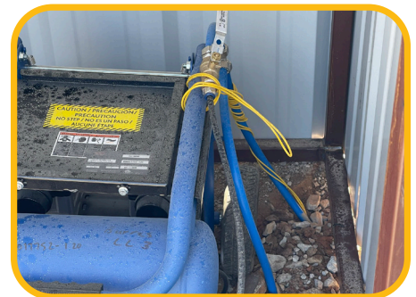
MaxLine attached to air compressor
