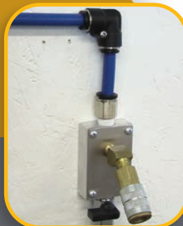
Surface Mount Air line is mounted to wall
